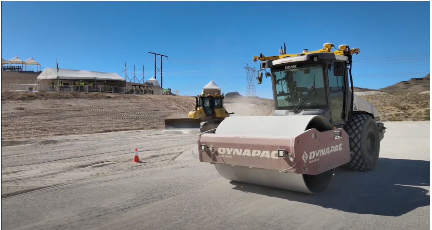
Trimble Autonomy enabled autonomous compactor shown at Dimensions 2022. Photo Credit: Matt Sewick
